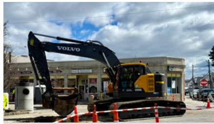
The Massachusetts Department of Transportation has announced that $45 million in supplemental funding for road and bridge repair and construction is available to communities.
