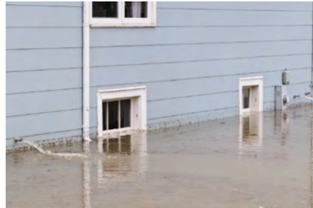
Municipalities can take a number of steps to help lessen the likelihood of costly damage resulting from floods.
