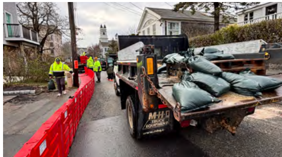
Provincetown Public Works staff install a new flood barrier during a test run last December.
