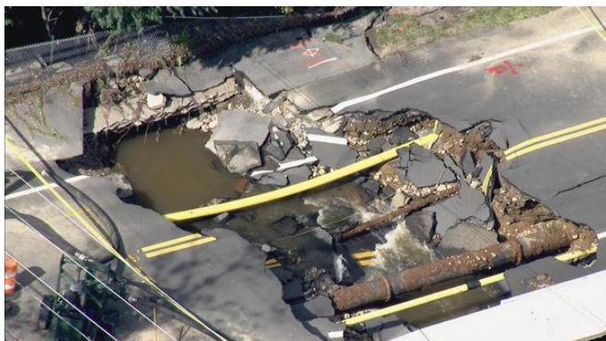
Photo 7: Washed out road in Leominster, following 10 inches in rain in six hours
